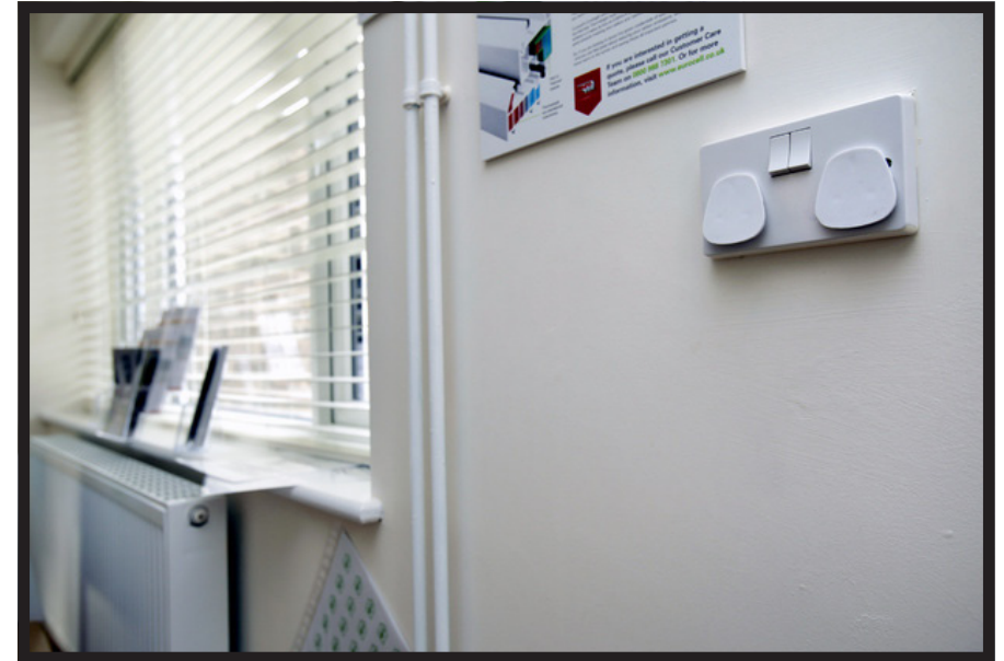
Elevated electrics and sockets © Huntingdonshire District Council
